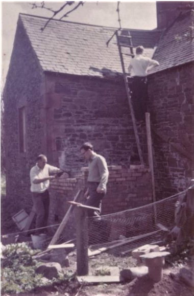
1966 – Drummonds Hall - the toilet block under construction - Peter Blythe, Gordon McConnachie, Allanach on ladder
